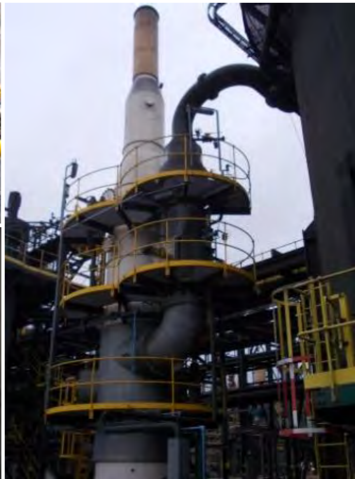
Venturi outlet: tangential inlet to cyclonic separator vessel
