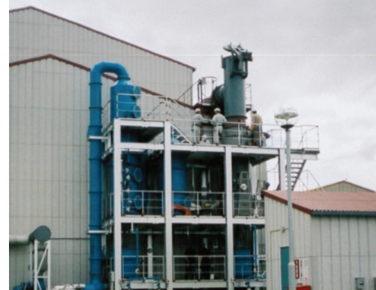
Flue gas treatment for precious metal recovery smelter, Japan
