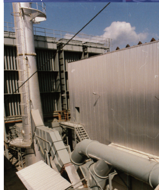
Zinc smelter reverberatory furnace flue gas treatment, Malaysia
