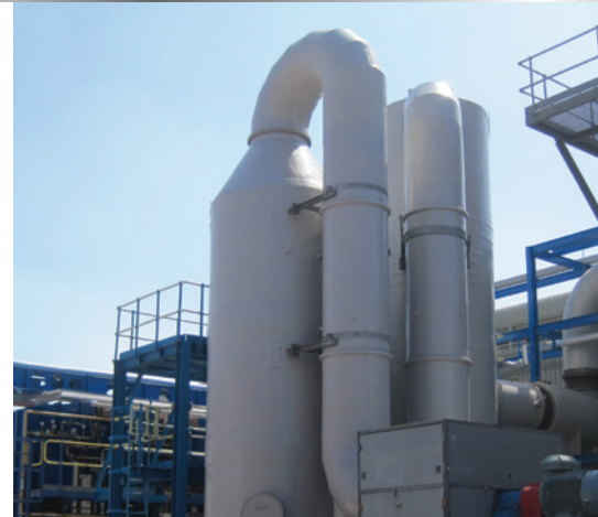
Flue gas treatment for manufacture of alumina based fibre, UK
